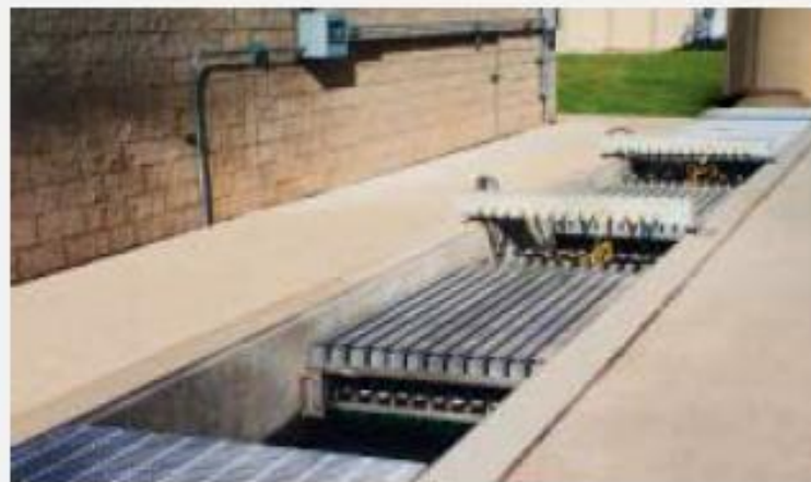
b. Open-Channel Reactor
